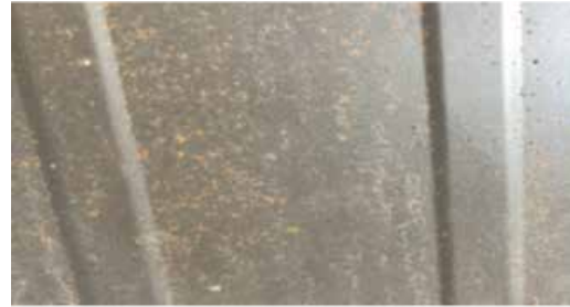
Heavy swarf staining on pre-painted steel.
